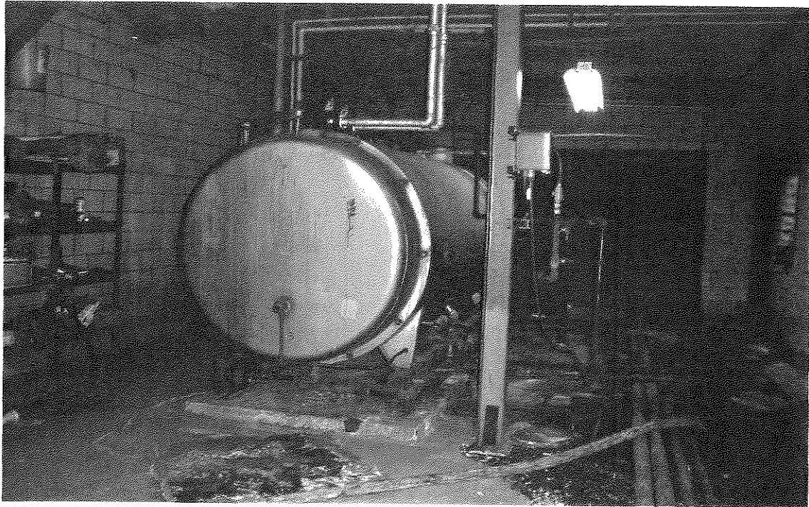
BECHTEL-MCLAUGHLIN (BOILER ROOM): ACTIVE BOILER
