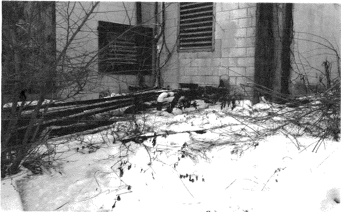
BECHTEL-MCLAUGHLIN: PIPING TO WATER TREATMENT
